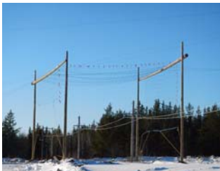
Photo courtesy of Manitoba Hydro
